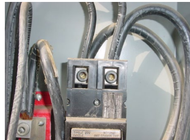
Double Tapped Wires
