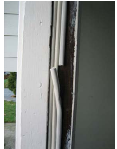
Weather stripping on doors prevents infiltration and loss of conditioned air from inside the home. Make sure your doors are properly sealed by inspecting the gasket material.
