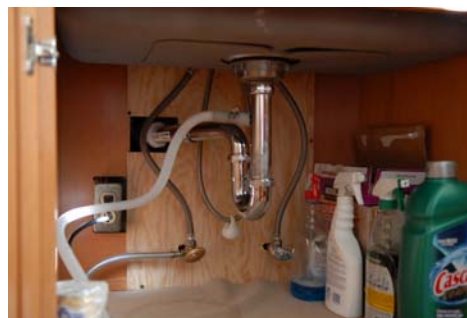
Inspect under sinks for wall penetrations made for plumbing and electrical systems. Sealing off these areas will reduce infiltration and keep conditioned air in the home where it belongs.
