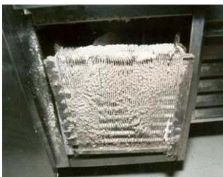
Poor filter maintenance or unfiltered return air will contaminate a condensing coil making it difficult for equipment to function. This unit will require a professional cleaning costing hundreds of dollars. In the long run proper filter maintenance is cheaper!
