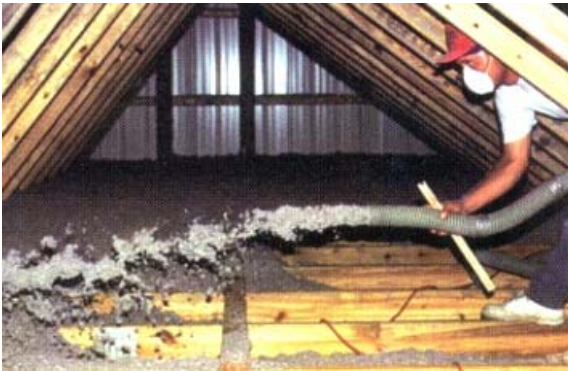
Attic insulation slows heat loss in the winter and stops heat gain in the summer. Insulation and proper attic ventilation are important for comfort and efficiency.
